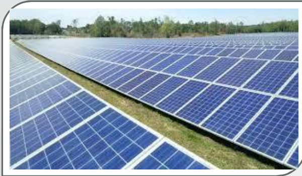
Solar PV Panels
